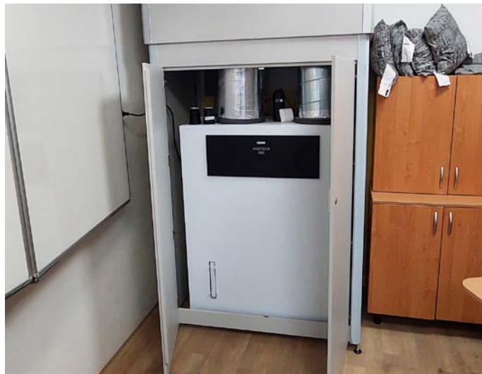
Installed VENTBOX 800 unit in one of the classrooms
